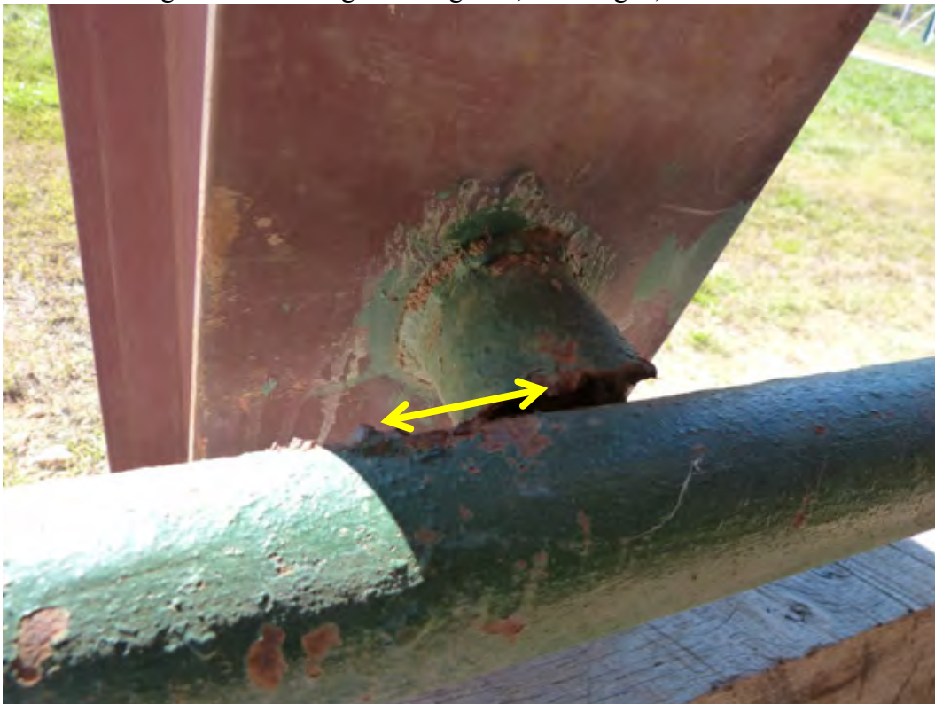
Figure 18 – Damaged G5R girder, Building C, sideways displacement.
