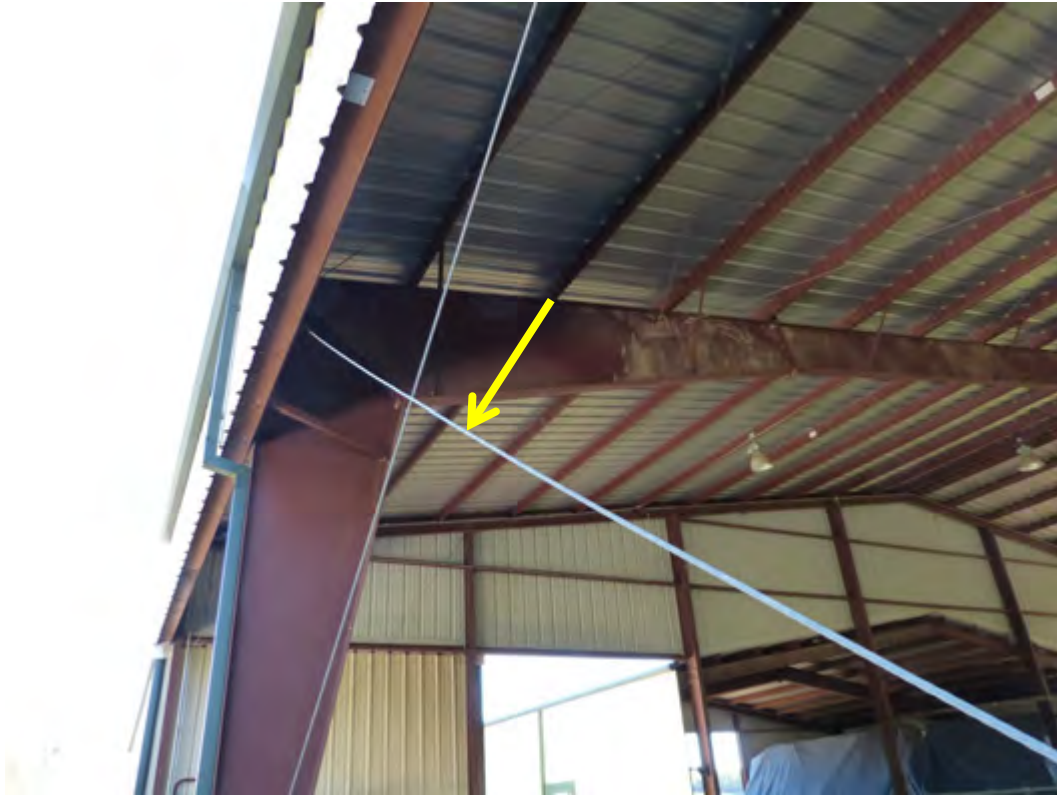
Figure 19 – Loose sidewall cable bracing, Building C, North side.
