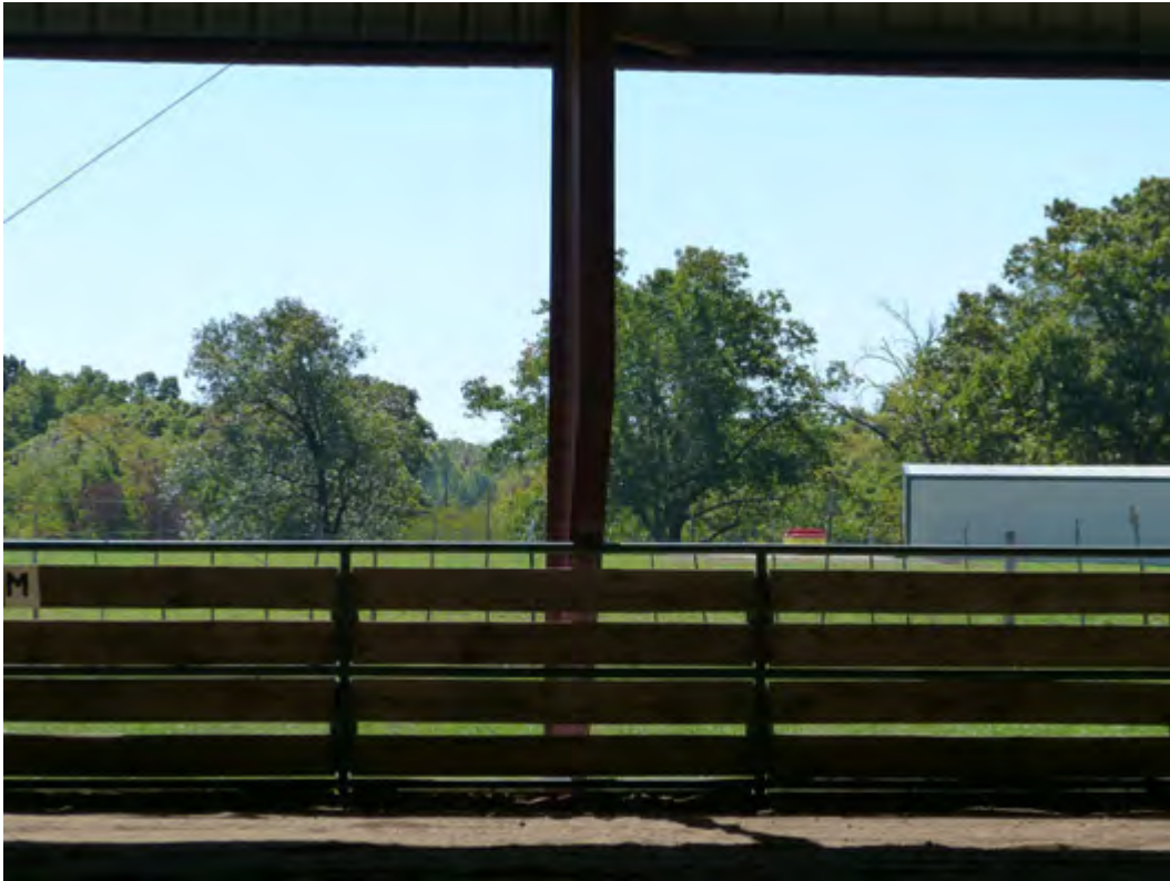
Figure 17 – Damaged G5R girder, Building C, inside view.
