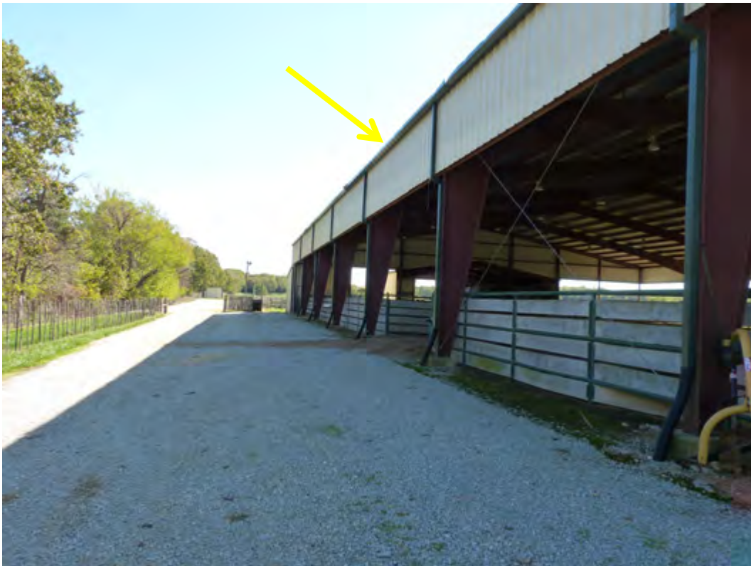
Figure 2 – Damaged gutter Building C, North side
