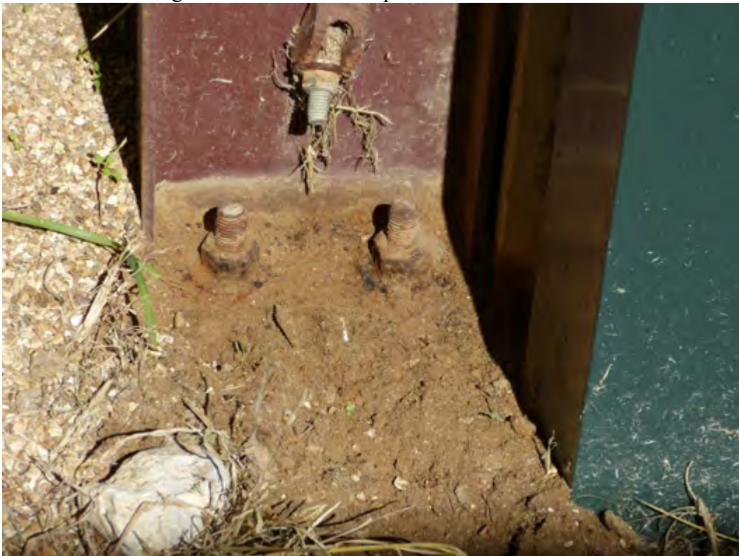
Figure 26 – Rusty bolts in Figure 25 exposed.
