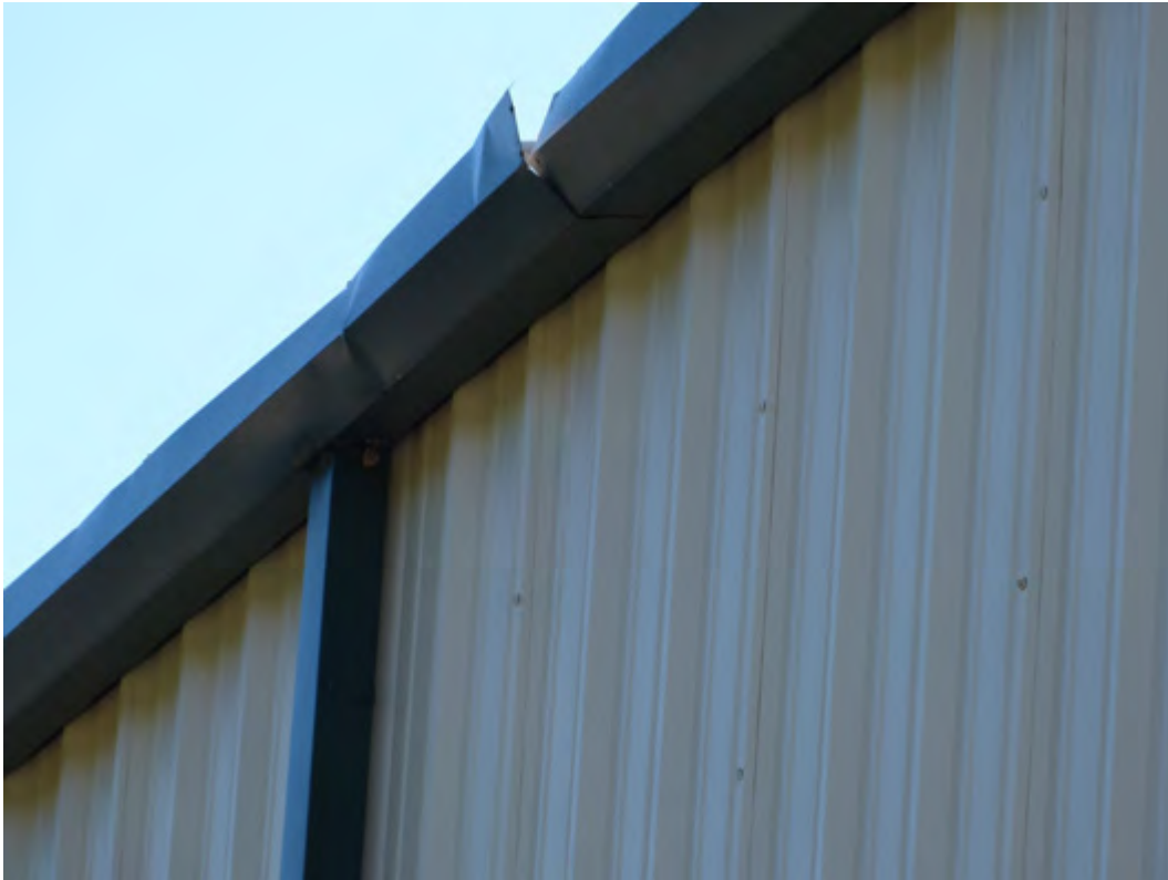
Figure 3 – Close-up view of damaged gutter in Figure 2
