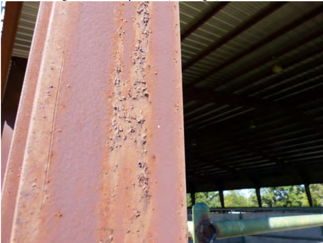
Figure 24 – Surface rust on exposed structural steel.
