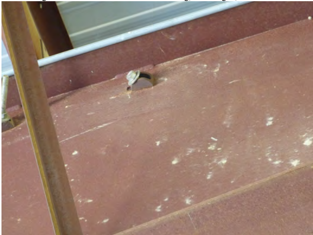
Figure 20 – Roof cable bracing eye-bolt nut
