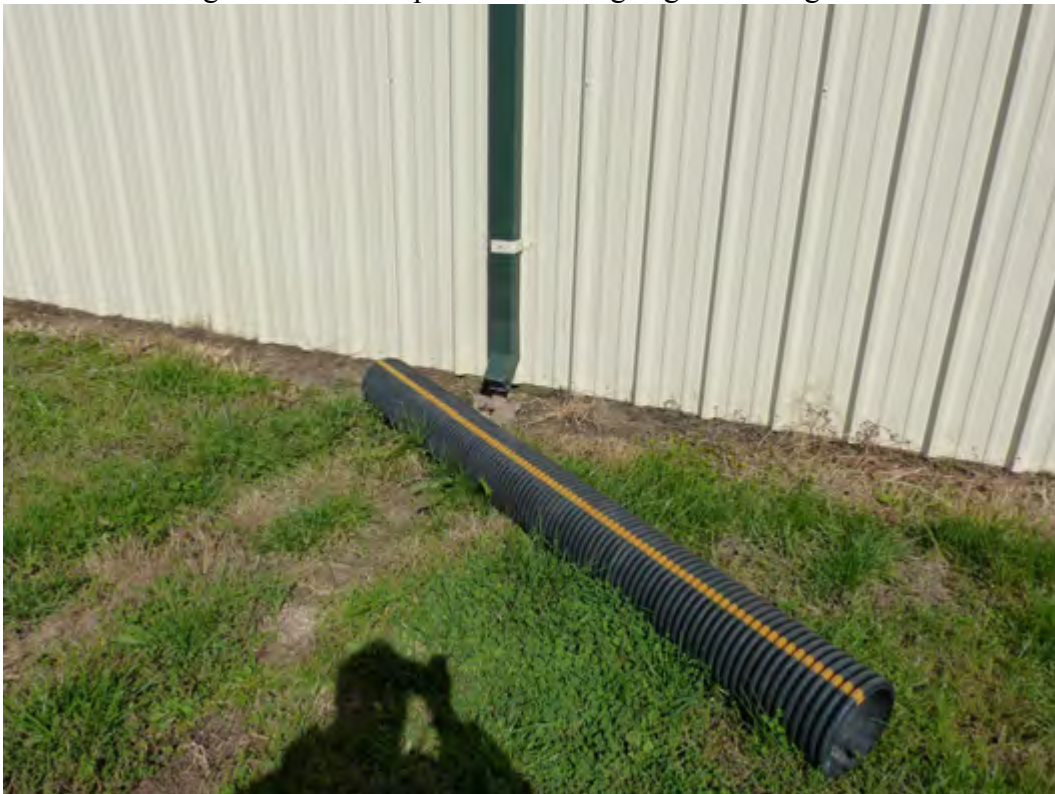
Figure 6 – Downspout discharges next to foundation, South side of Building D
