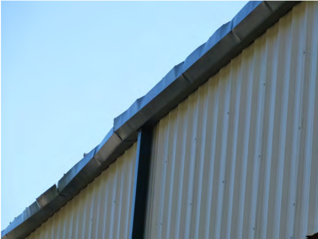
Figure 5 – Close-up view of damaged gutter in Figure 2
