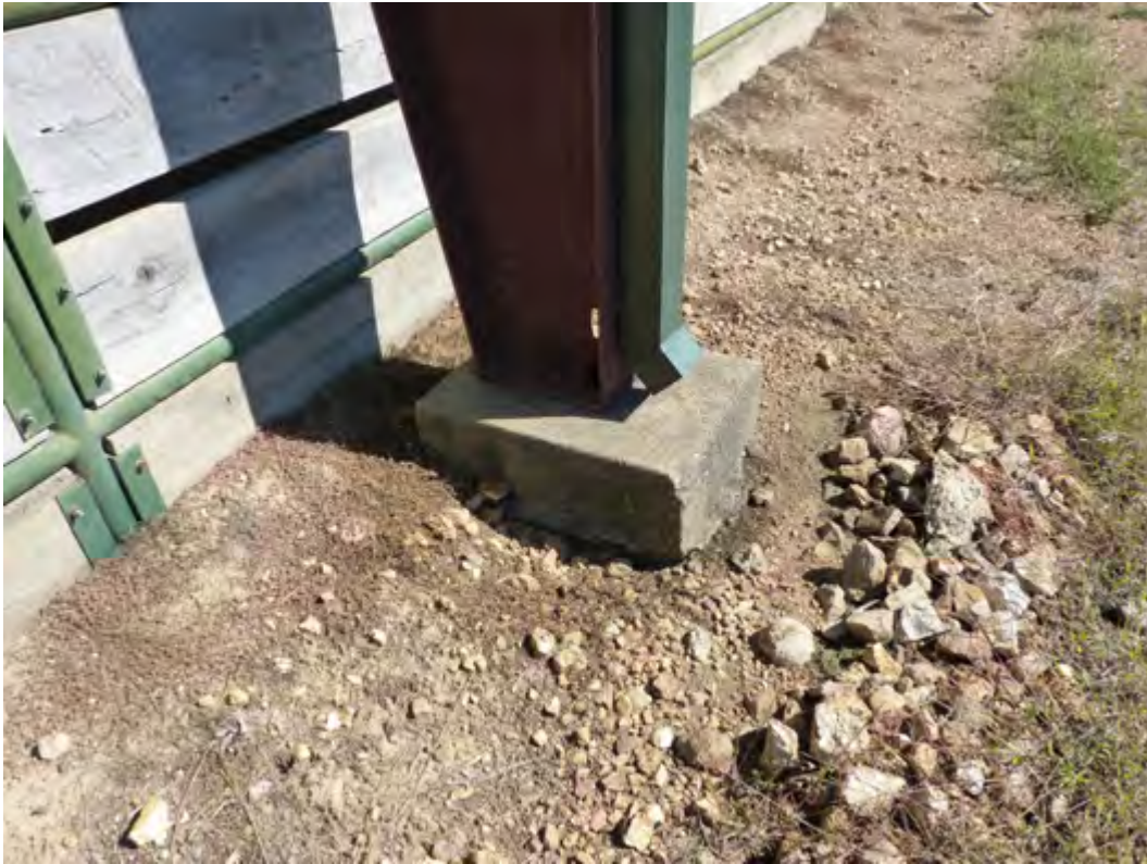
Figure 11 – Footing at girder G4R, Building C, South side.
