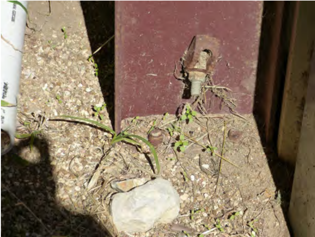
Figure 25 – Column base plate covered with soil.
