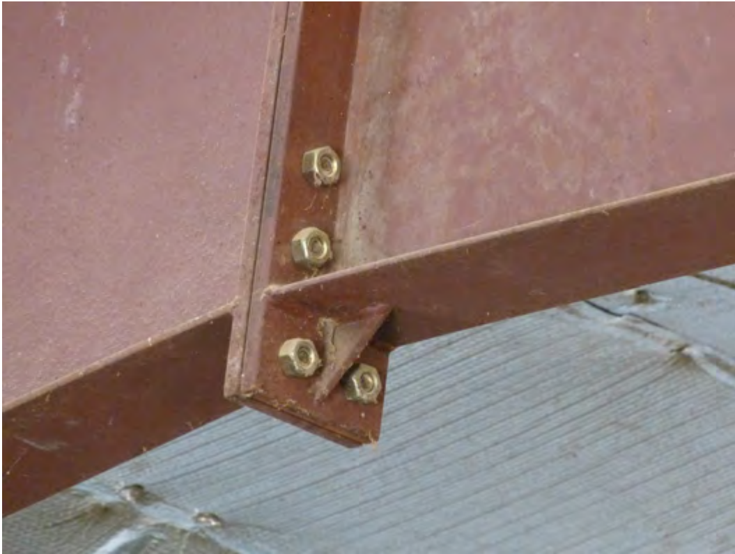
Figure 23 – Short splice bolts, Building B, center beam.
